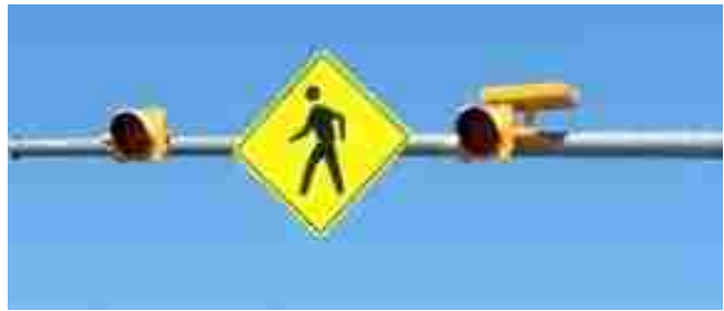
(b) Circular Rapid Flashing Beacons (CRFB)
