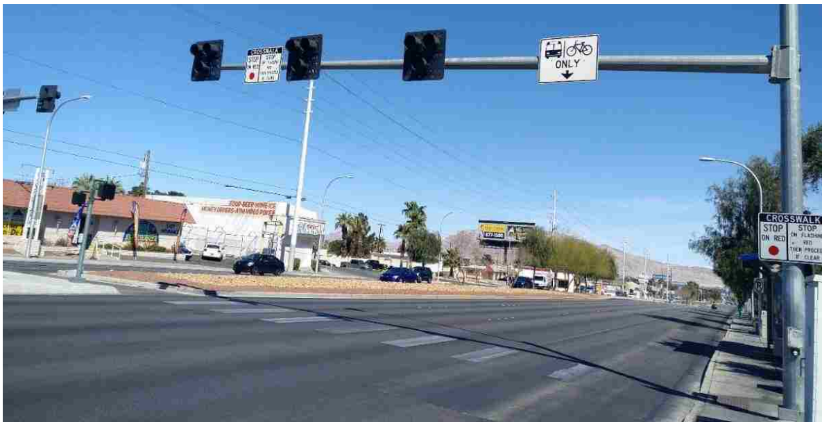
Figure 7. Installed Pedestrian Hybrid Beacons (PHBs)
